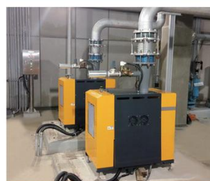
河北沧州化工厂 Cangzhou Hebei chemical plant
