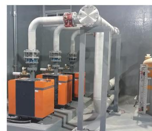
四川乐山污水处理厂 Leshan Sichuan sewage treatment plant
