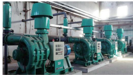
大庆肇源污水处理厂 Zhaoyuan Daqing sewage treatment plant
